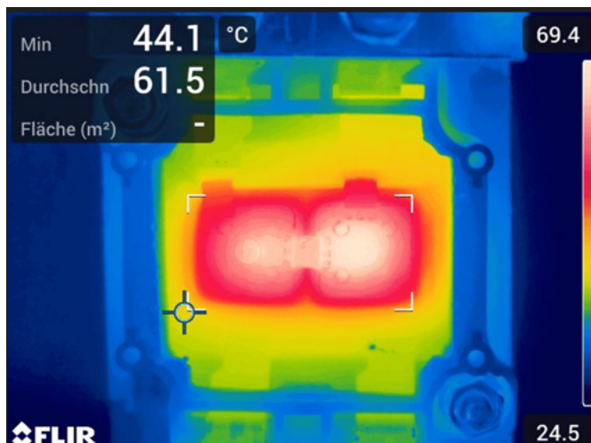
Figure 1: IR image of two diodes connected in parallel under DC load
