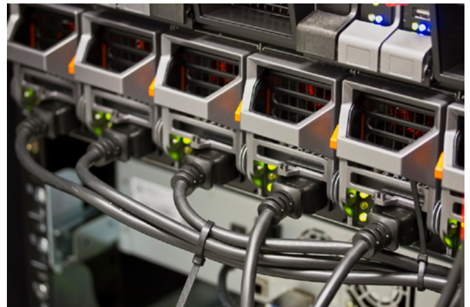
Figure 2: Modern data centers require huge amounts of power
