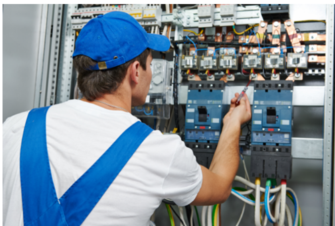
Figure 1: Mersen-ProGrid-building-distribution-Adobe-Stock_491977888.jpg: Smart fuse switch disconnectors from Mersen monitor the current flow in building distribution systems (Image: ©stock.adobe.com/Kadmy)
